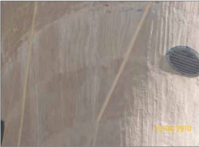
Water leakage and corrosion damage prior to restoration
