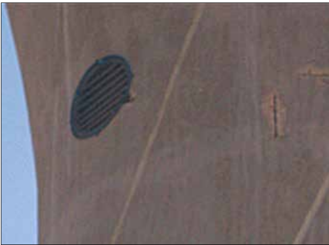
Corrosion damage prior to restoration
