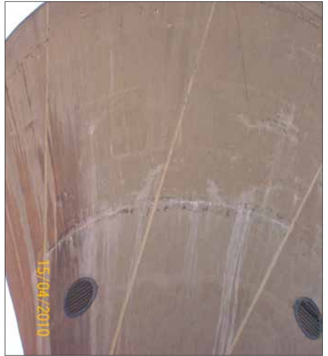
Water leakage and corrosion damage prior to restoration
