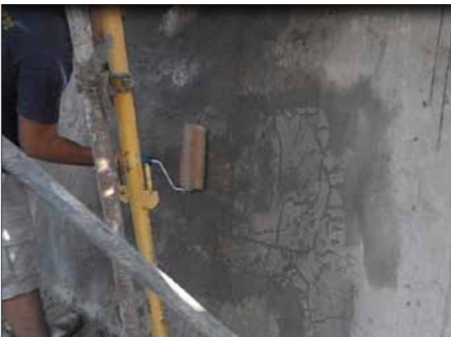
Roller application of MCI®-2020 was chosen as wind around high exposed tower may carry spray droplets
